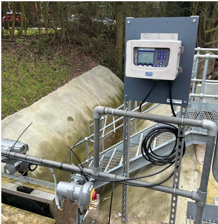
Teledyne ISCO's Signature flow meter is installed above the discharge channel and receives data from the 350Ex sensor.
